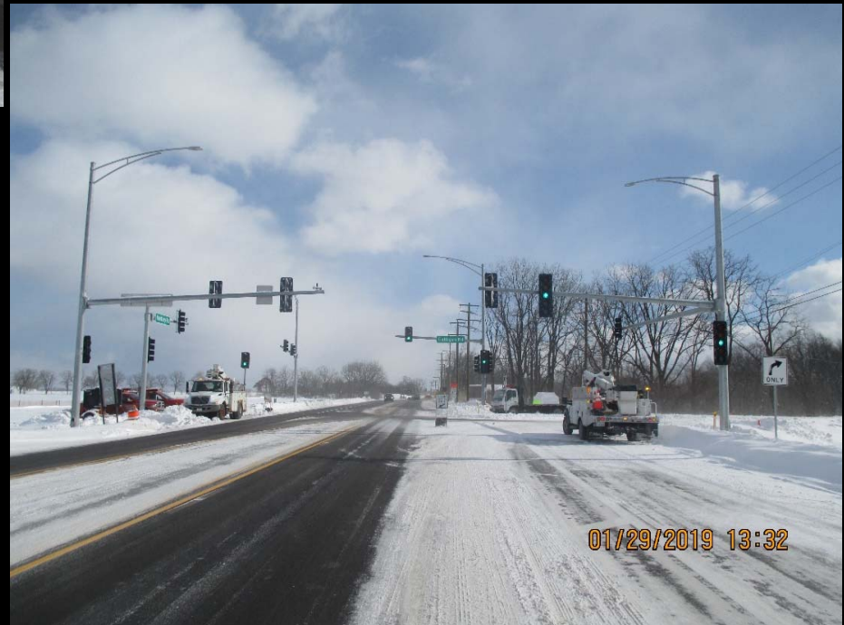
Crews test and activate the new signals on the Huntley Rd at Galligan Rd Intersection Improvement
