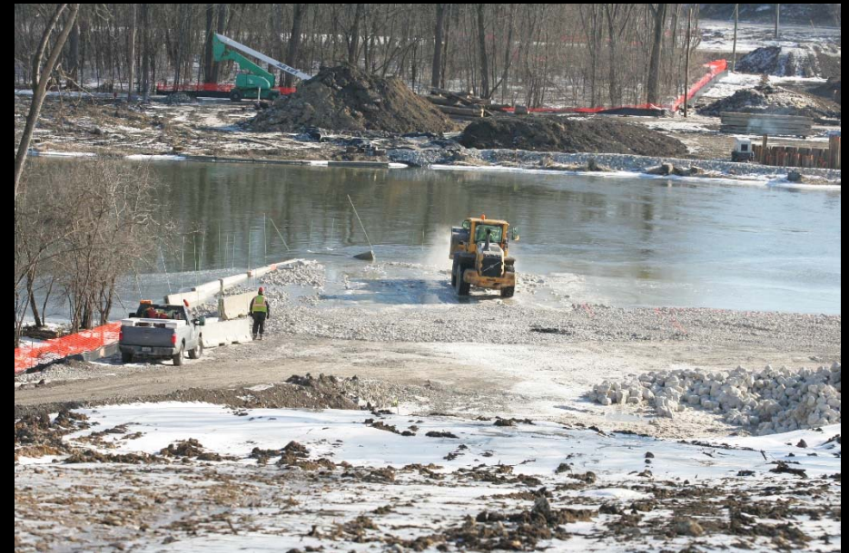
Crews work on the causeway in order to start pier work for the LMP C1- East of IL 31 to Sandbloom Road project
