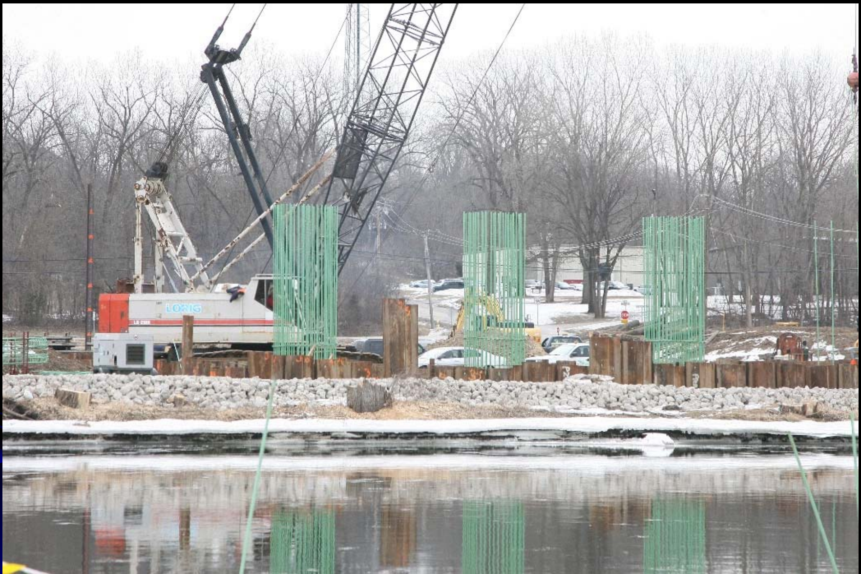
Working in-between the freeze spells the contractor places reinforcing bars for the piers for the LMP C1- East of IL 31 to Sandbloom Road project
